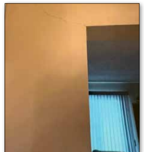
Cracking in the drywall appeared throughout the home following the seismic activity in the area.
