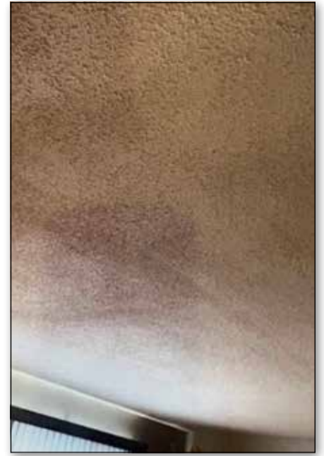
Sagging drywall in the living room ceiling is among the damage Sturgeon County resident Peter Pedgerachny says was caused by a series of earthquakes felt throughout the region earlier this spring.
