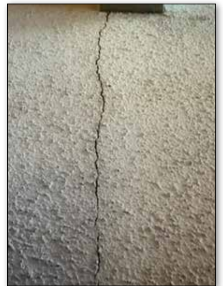
A large crack in the ceiling is one of several areas of damage found throughout the home after the earthquakes.
