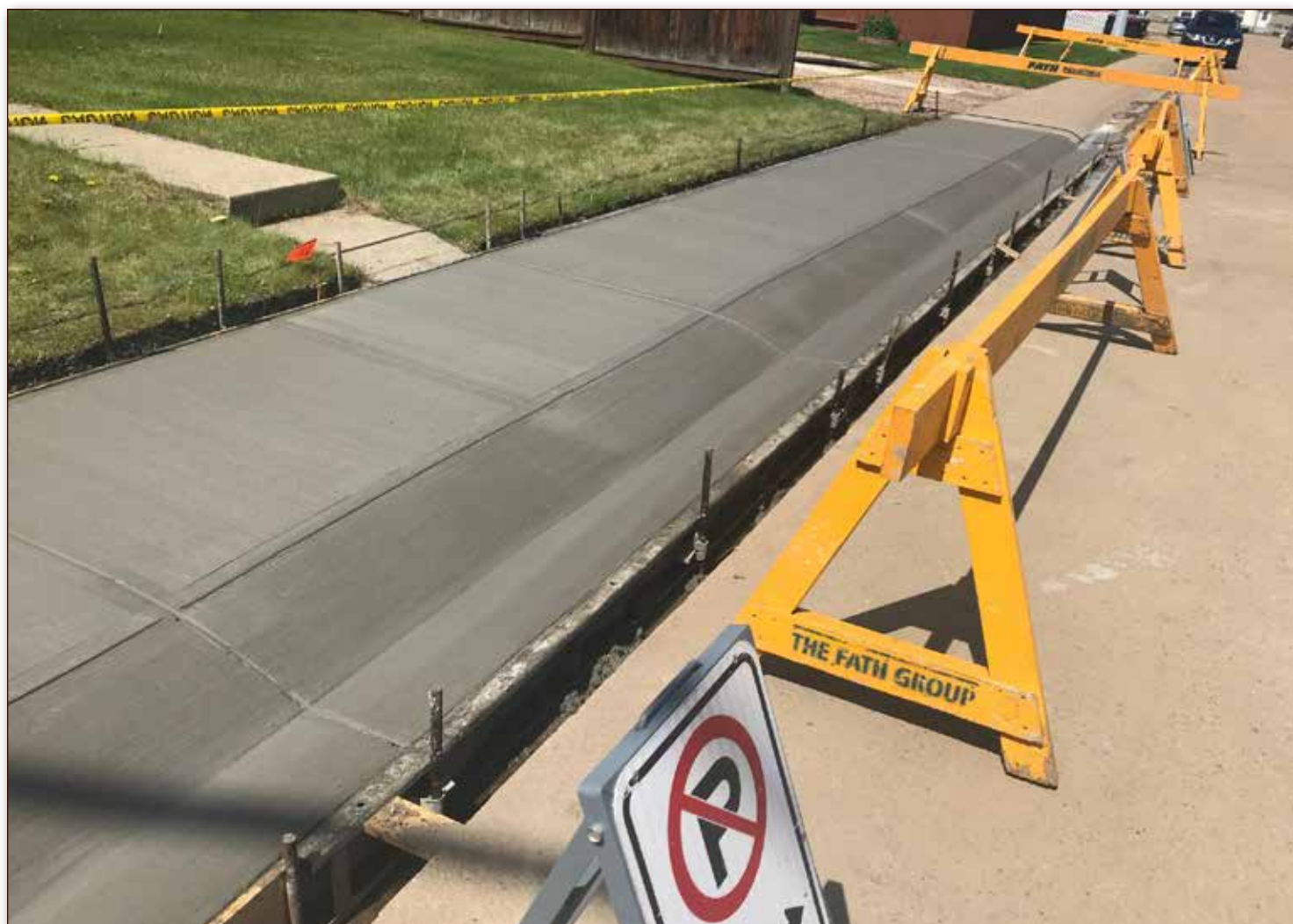
It's that time of year again when the annual sidewalk replacement program begins! The program began July 15 and will continue for a couple of weeks. O'Hanlon Paving will be around the Town of Redwater to remove and replace sidewalks, so please watch out for barricades and signage. If you have any further questions or comments, fill out a service request to public works at: http://www.redwater.ca/p/service-request or call the Town Office at 780-942-3519 Ext 290. Photo: Town of Redwater
