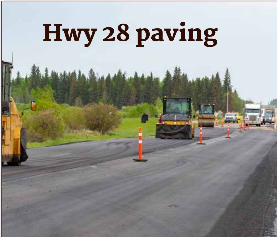
Heavy equipment operators with Ledcor Group pave Highway 28 south of Redwater on June 4. Road safety crews kept the traffic moving with minimal delays as paving crews worked to improve the highway. Photo by Grant Cree
