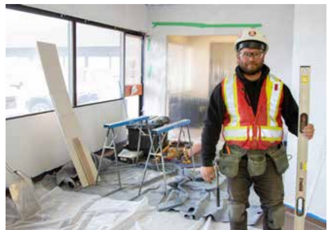
Jason Kilburn, Foreman with Cobra Contracting, stands in the Redwater Town Office reception area on April 21 during renovations. The Town office is scheduled to be open to the public in late April. Photo by Grant Cree
