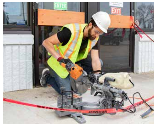
Adrien Gagnon with Cobra Contracting operates a radial mitre saw outside the Redwater Town Office on April 21 during renovations. The concrete sidewalk at this main entrance will be modified for wheelchair accessibility. The Town office is scheduled to be open to the public in late April. Photo by Grant Cree
